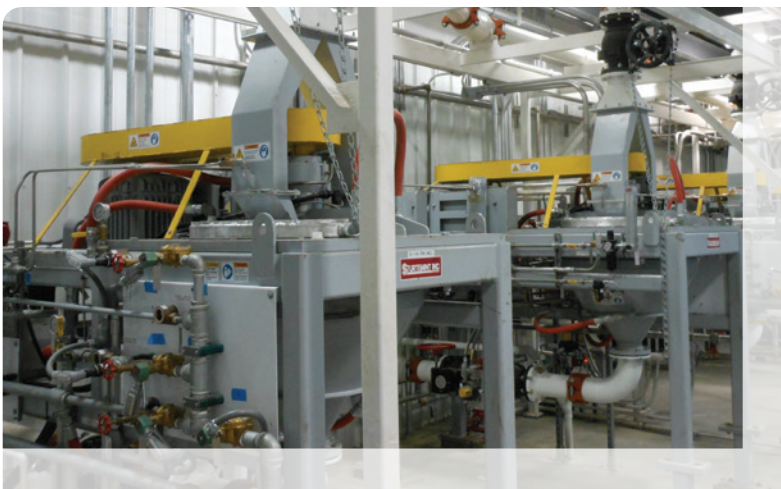
Trona mill system installed at a coal fired power plant.
