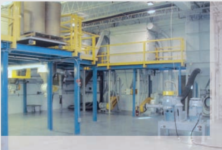
Sturtevant's test facility
