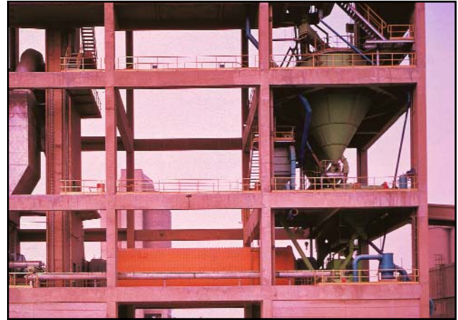
16-foot Whirlwind installed in grinding circuit producing 325 mesh product
